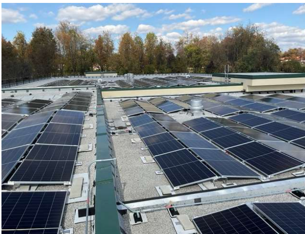
5 - ROOF WITH SOLAR PANELS
