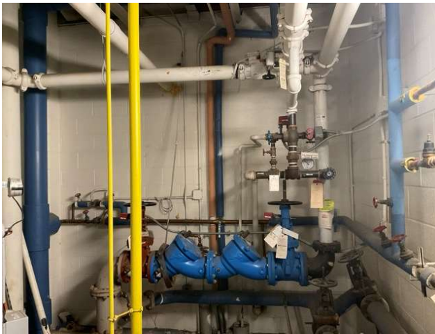
33 - FIRE SUPPRESSION SYSTEM
