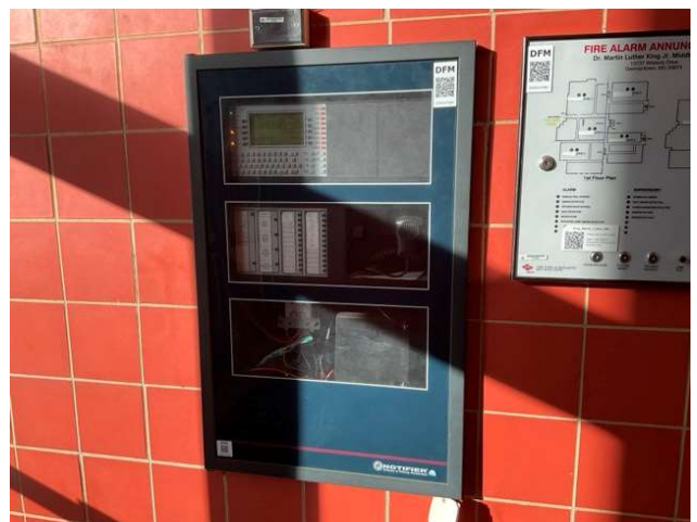
36 - FIRE ALARM PANEL
