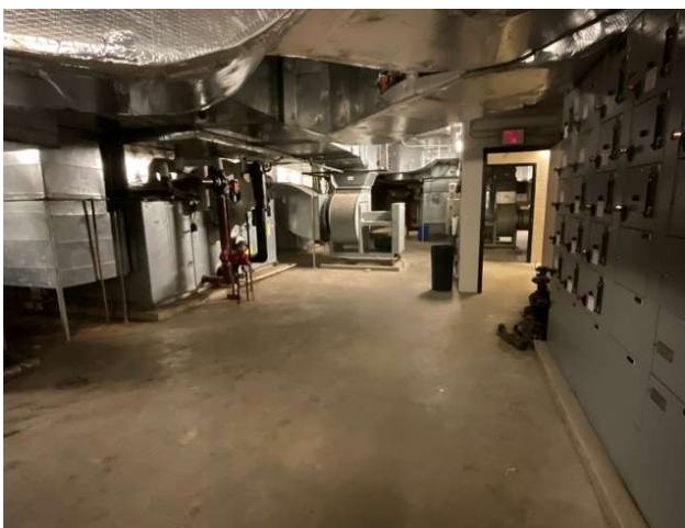
29 - PENTHOUSE MECHANICAL ROOM
